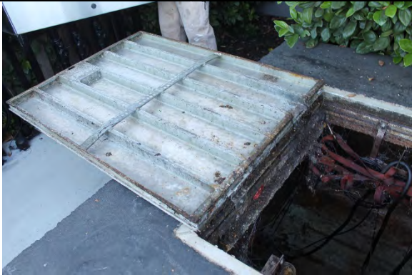
Wet well hatch in poor condition.
