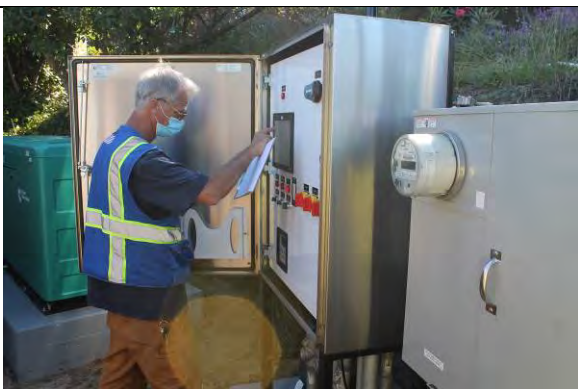
Electrical and I&C upgraded in 2017 and in very good condition.
