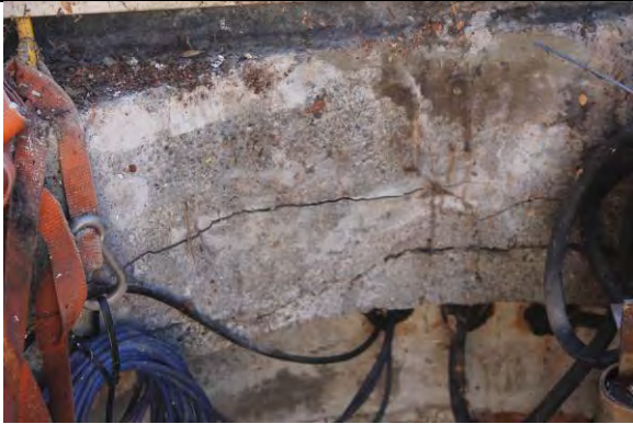
Wet well grout exhibiting cracking.
