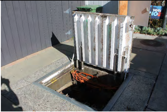
Painted wet well steel access hatch is in good condition and exhibiting light surface corrosion.
