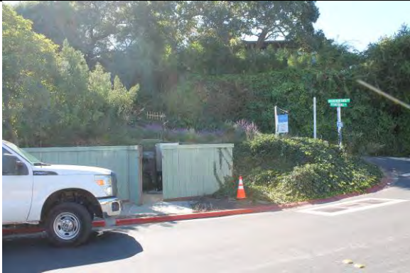
Lift station in good to poor condition. Odor issues reported. Previously had Bioxide odor control injection but was removed during the new backup generator installation. Instead currently using manhole odor control inserts for odor control. However, the Bioxide system is preferred.
