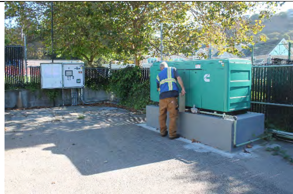
Recently upgraded natural gas backup generator.
