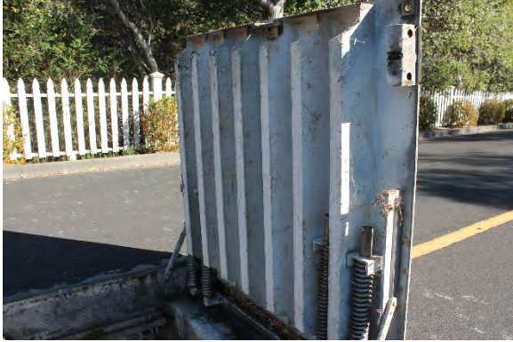
Painted wet well steel access hatch is in good condition and exhibiting light surface corrosion.
