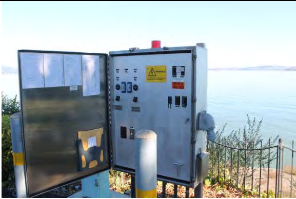
Electrical and I&C upgraded in 2009 and is in good condition.
