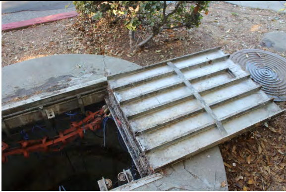
Wet well access hatch in fair condition and concrete top cracked and in poor condition.
