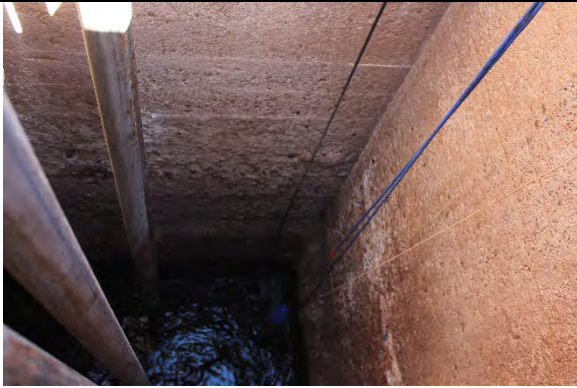
Wet well concrete in poor condition and exhibiting exposed aggregate, softness, and H 2 S corrosion.
