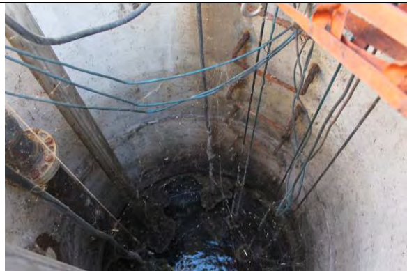
Wet well concrete is in fair condition. Access ladder is in very poor condition, extremely corroded, and should not be used.
