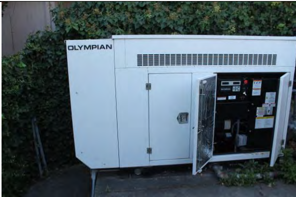
Generator upgraded recently and provides backup power to Tiburon 1 and 2.
