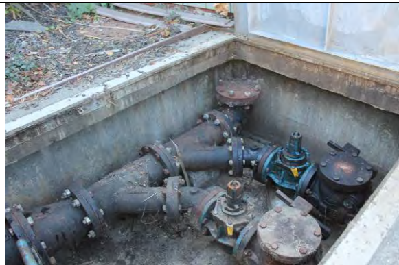
Valve vault concrete and hatches in fair condition. Isolation and check valves are in fair to poor condition.
