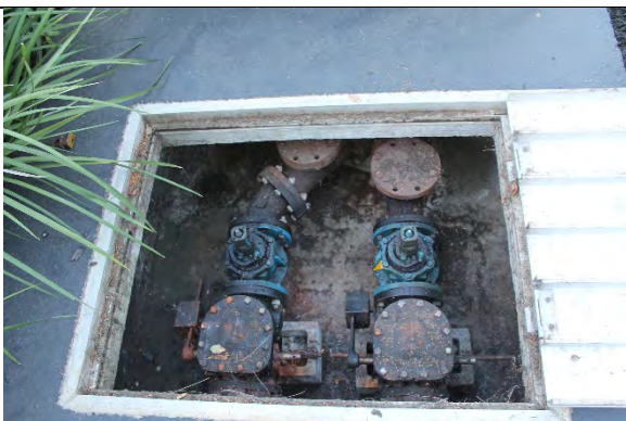
Isolation and check valves in fair and poor condition, respectively. Check valves were stuck.
