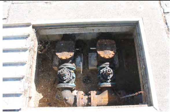
Isolation and check valves in fair and poor condition, respectively. Check valve issues reported.
