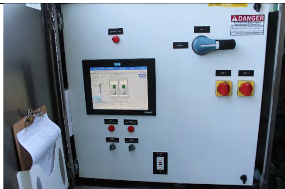
Electrical and I&C recently upgraded. Backup power provided by portable generator.
