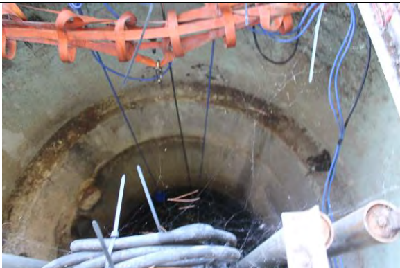
Wet well grout cracking and in fair condition.
