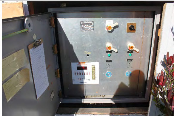
Older I&C scheduled to be upgraded.
