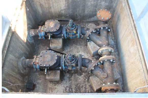
Isolation and check valves are in fair and poor condition, respectively.
