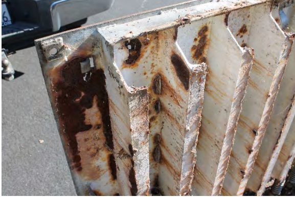
Painted wet well steel access hatch is in fair condition and exhibiting moderate surface corrosion.
