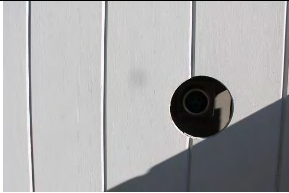
Pigtail for portable backup generator.
