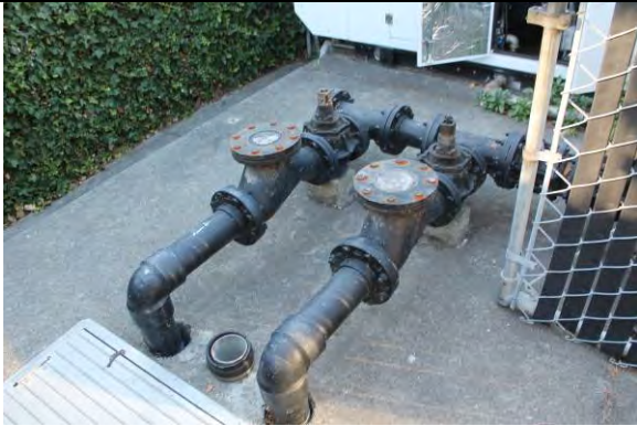
Check valves have not been upgraded.
