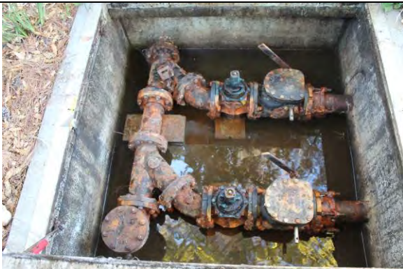
Standing water in valve vault causing piping surface corrosion. Isolation and check valves are in fair and poor condition, respectively.
