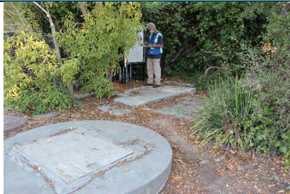
Wet well concrete top cracked and in poor condition.
