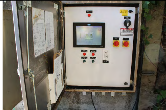
Electrical and I&C upgraded in 2015. Backup power provided by Tiburon 3 generator.
