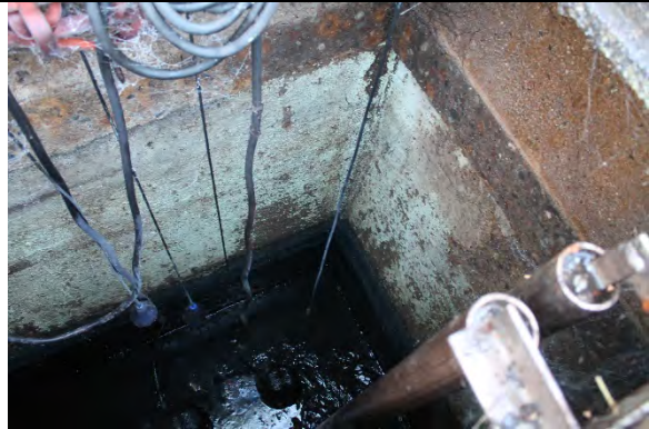
Wet well concrete in poor condition and exhibiting exposed aggregate and H 2 S corrosion. Previously painted.
