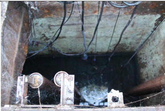
Wet well concrete in poor condition and exhibiting exposed aggregate and H 2 S corrosion. Previously painted.
