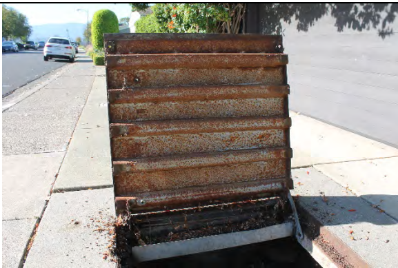
Valve vault steel access hatch is in fair condition and exhibiting moderate surface corrosion.
