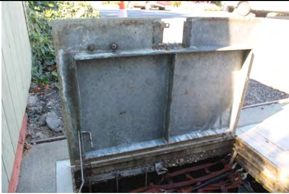
Wet well access hatches in fair condition exhibiting corrosion.
