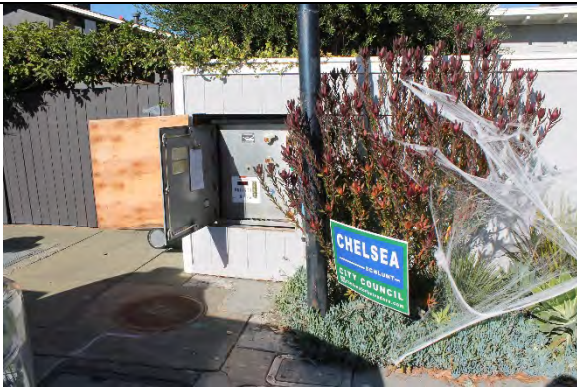
Lift station in fair condition. No access issues.
