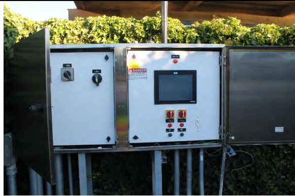
Electrical and I&C upgraded recently.
