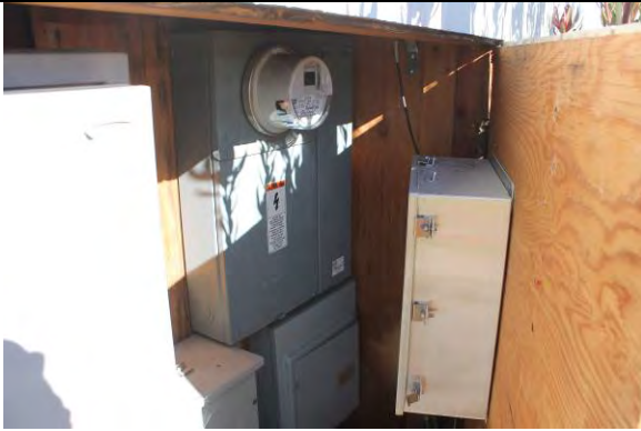
PG&E meter and circuit breaker panel.
