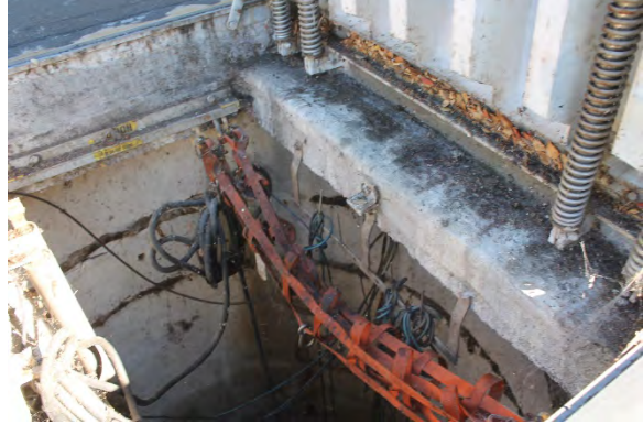
Wet well grout cracking and is in fair condition.
