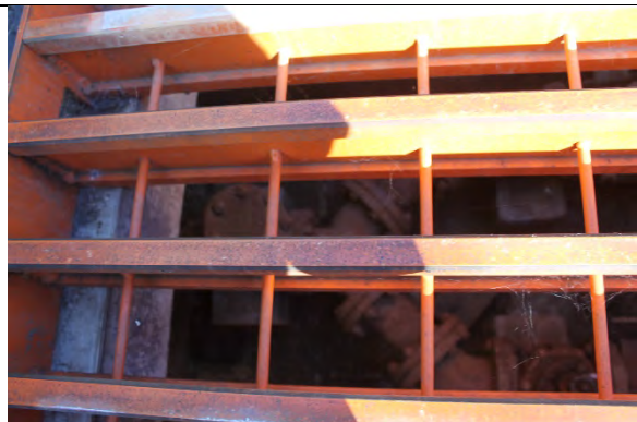
Fall protection safety grate in very good condition. Isolation and check valves are in good condition.
