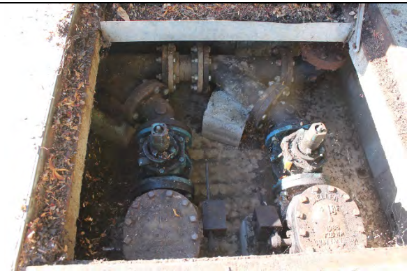
Valve vault concrete in fair condition. Isolation and check valves in fair to poor condition, respectively.
