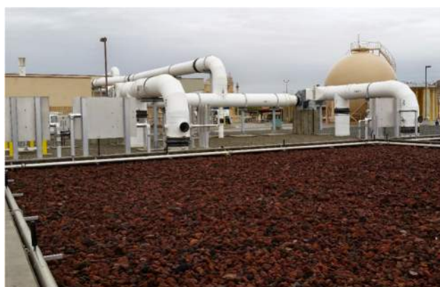
Below Ground Biofilter
