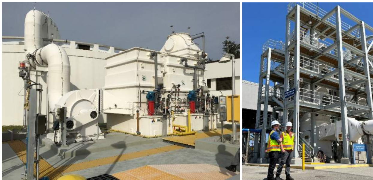
Figure 8 Chemical Scrubber System (Low Profile and Vertical Tower) Installations
