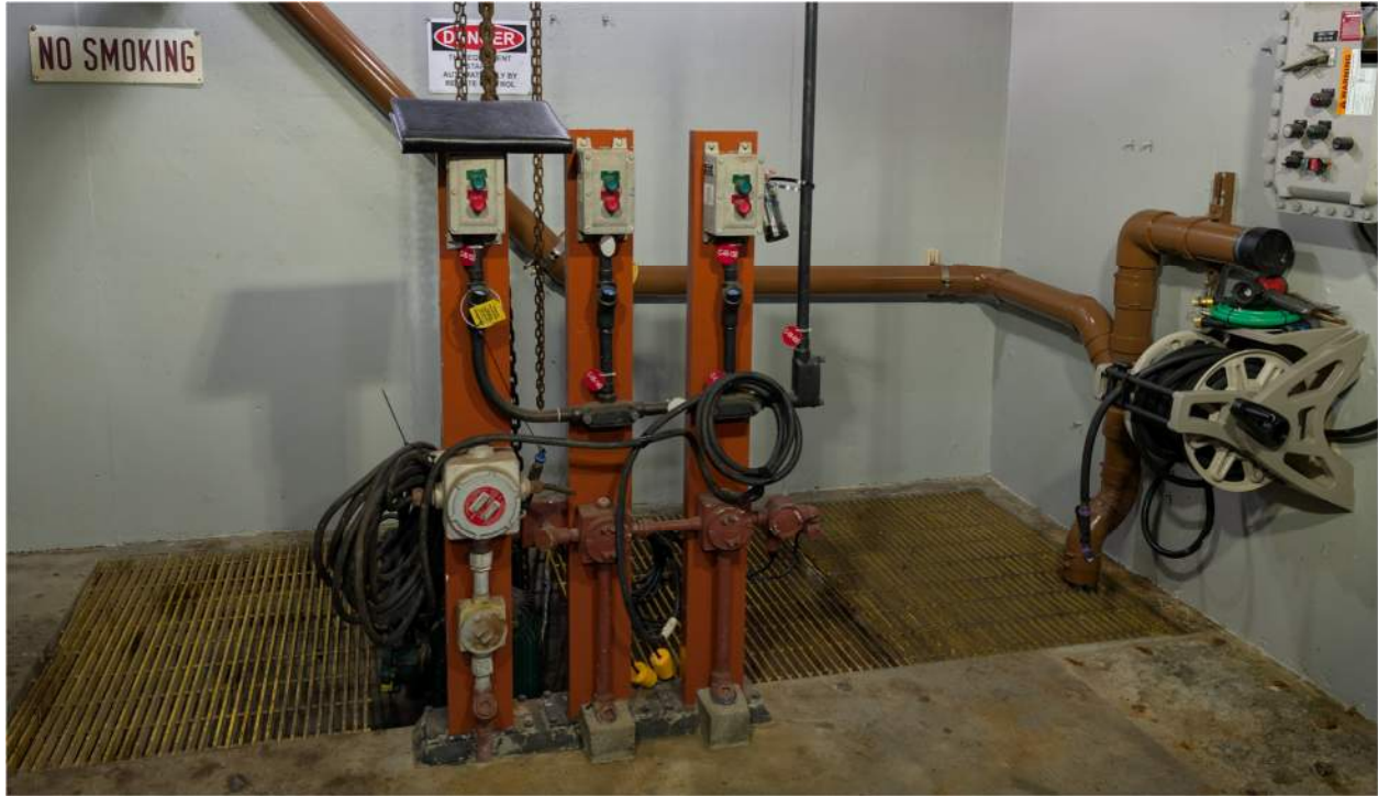
Figure 2 Sampling Location 2 – Headworks Inlet Room
