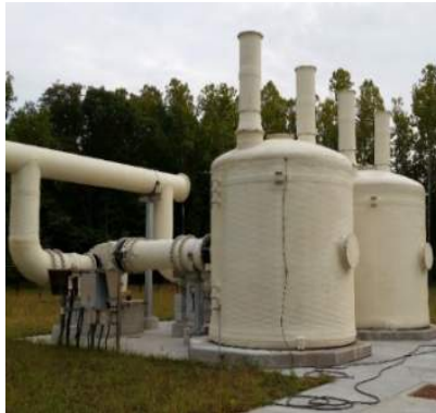
Dual Bed Carbon Scrubber
