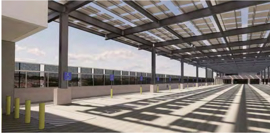
Figure 11 – Example, Canopy Mounted PV System
