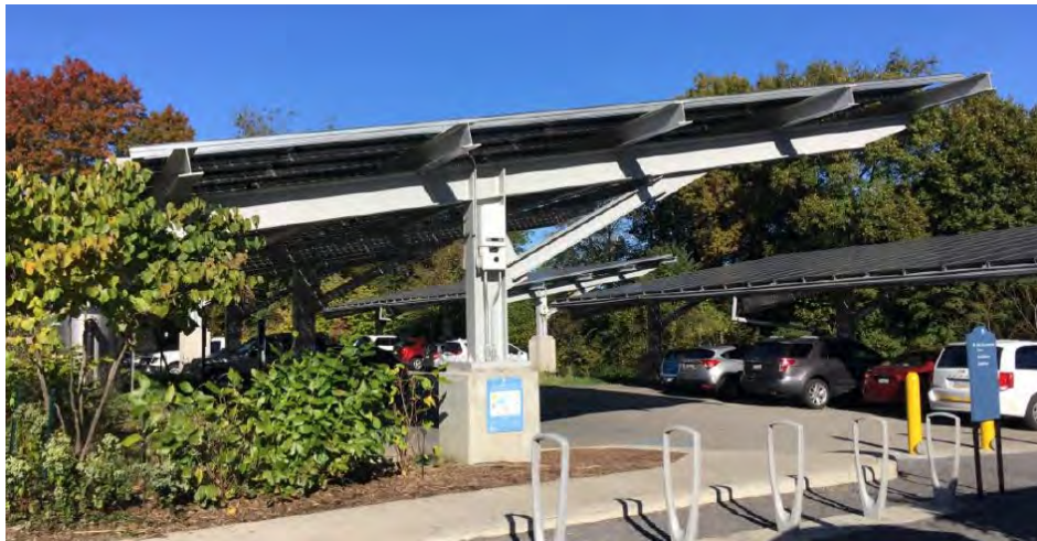
Figure 12 – Example, Carport Mounted PV System
