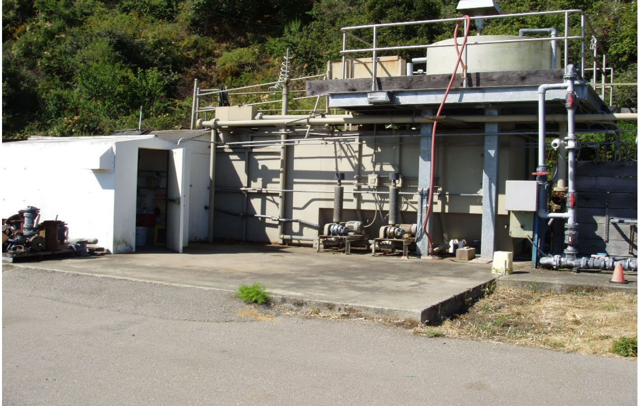
1980's era Unincorporated East Tiburon -Paradise Cove Wastewater Treatment Plant
