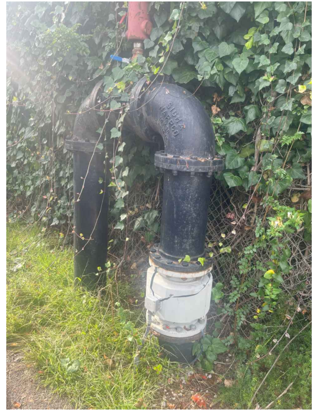
EXISTING FORCE MAIN FLOW TUBE
