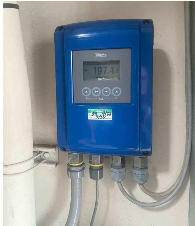
EXISTING PUMP FLOW TRANSMITTER
