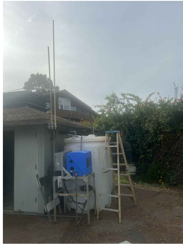
EXISTING CHEM PANELS & ANTENNAS
