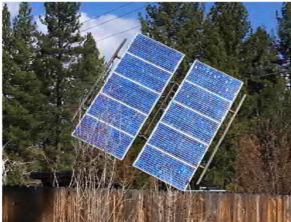
Figure 12 – Example, Active Tracking PV System
