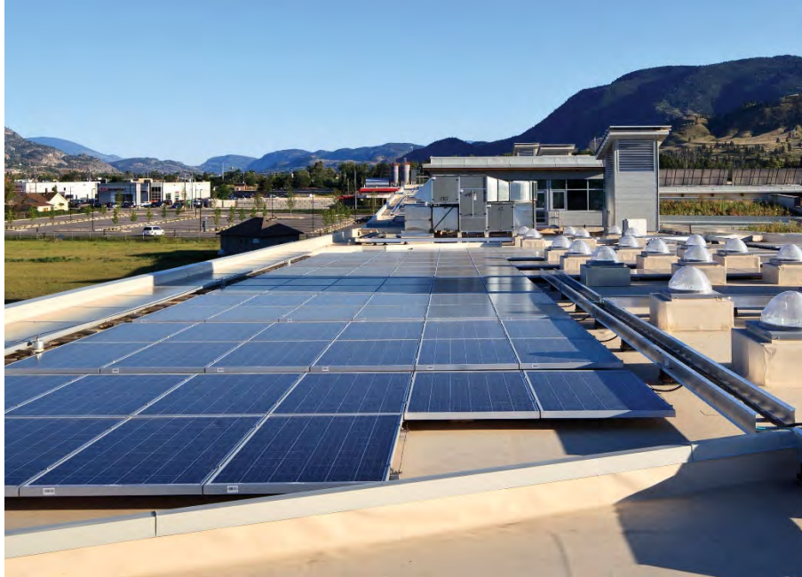
Figure 8 – Example, Roof Mounted PV System
