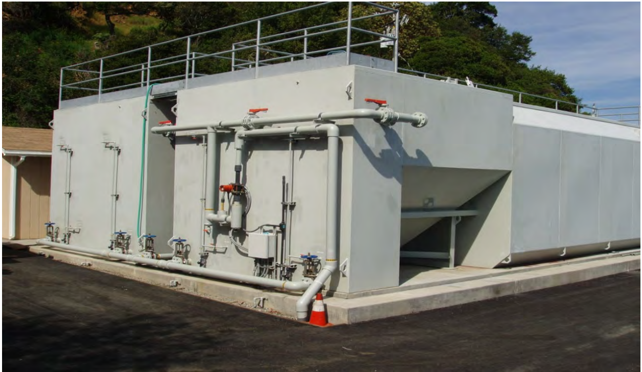
2010 Unincorporated East Tiburon- Upgraded Paradise Cove Wastewater Treatment Plant
